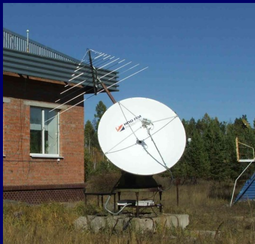
Antenna attached to dish
